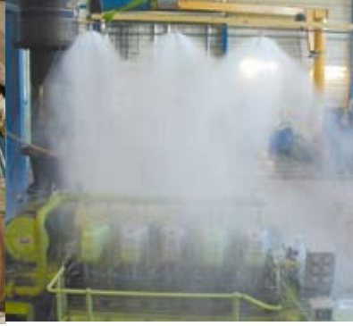
Diesel generator, Denmark
