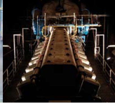
Diesel engine, Germany
